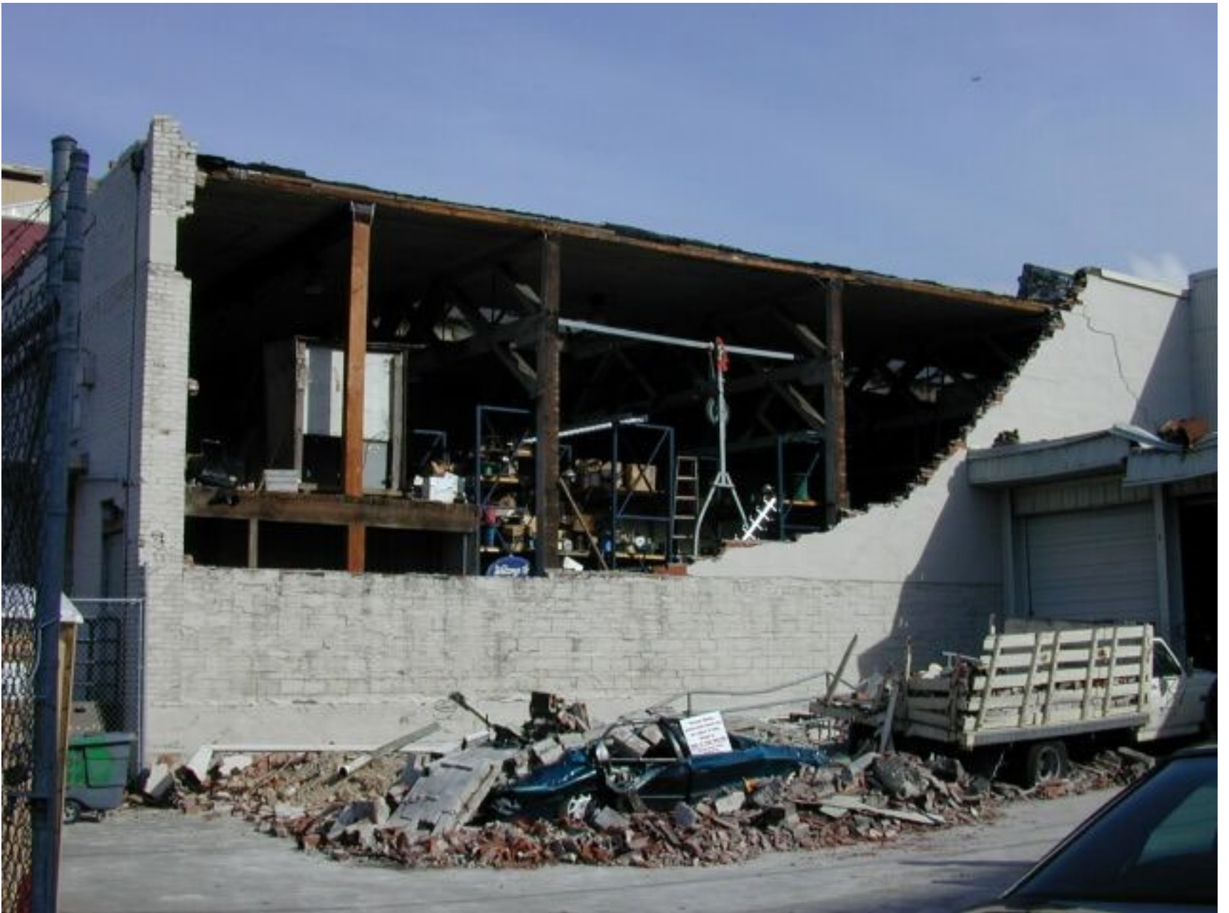
2001 Nisqually -- Collapsed URM, Seattle, Utah Avenue
